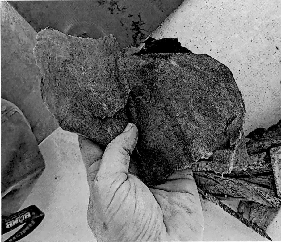
Figure 12 remnants of the paper face from the sheet rock.
