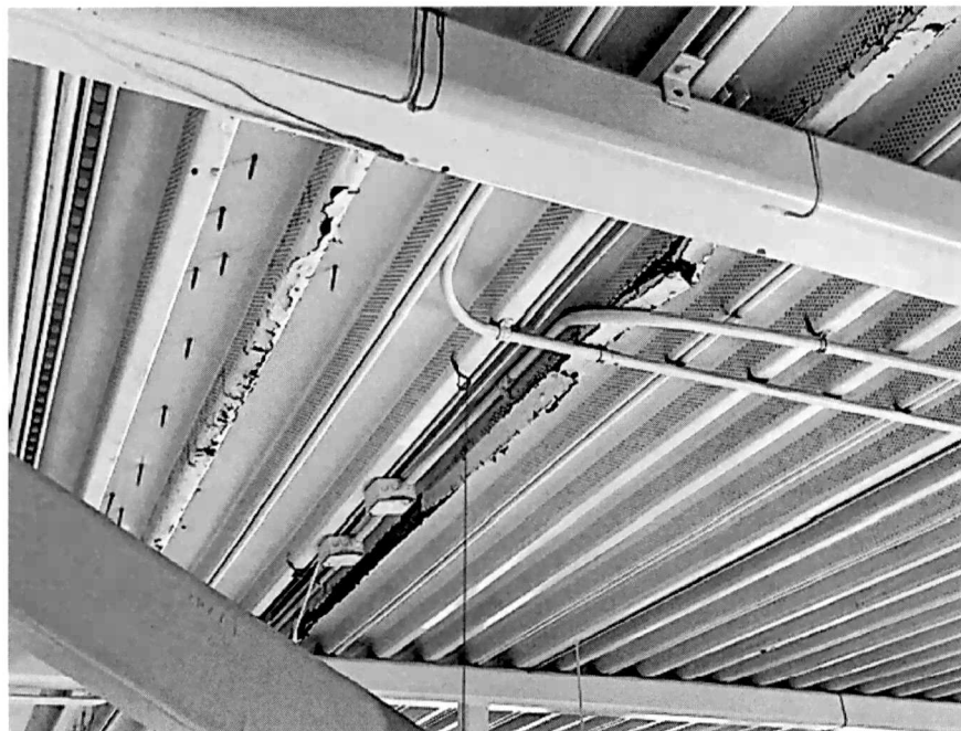
Photo-20: Severely damaged roof deck at north-west wall
