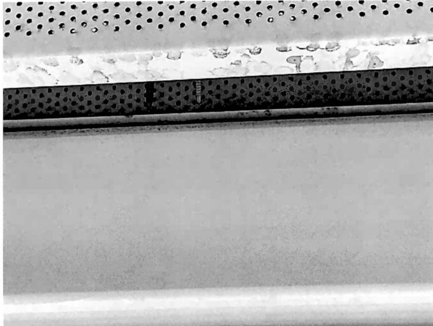
Photo-19: Lightly damaged roof deck bearing at south wall
