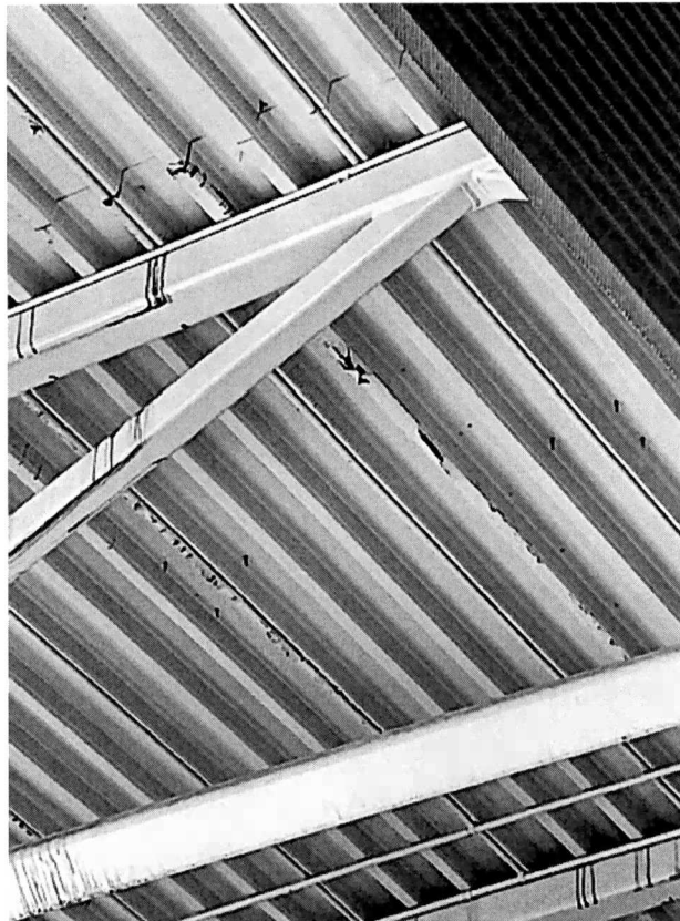
Photo-28: Severely damaged roof deck north of tower
