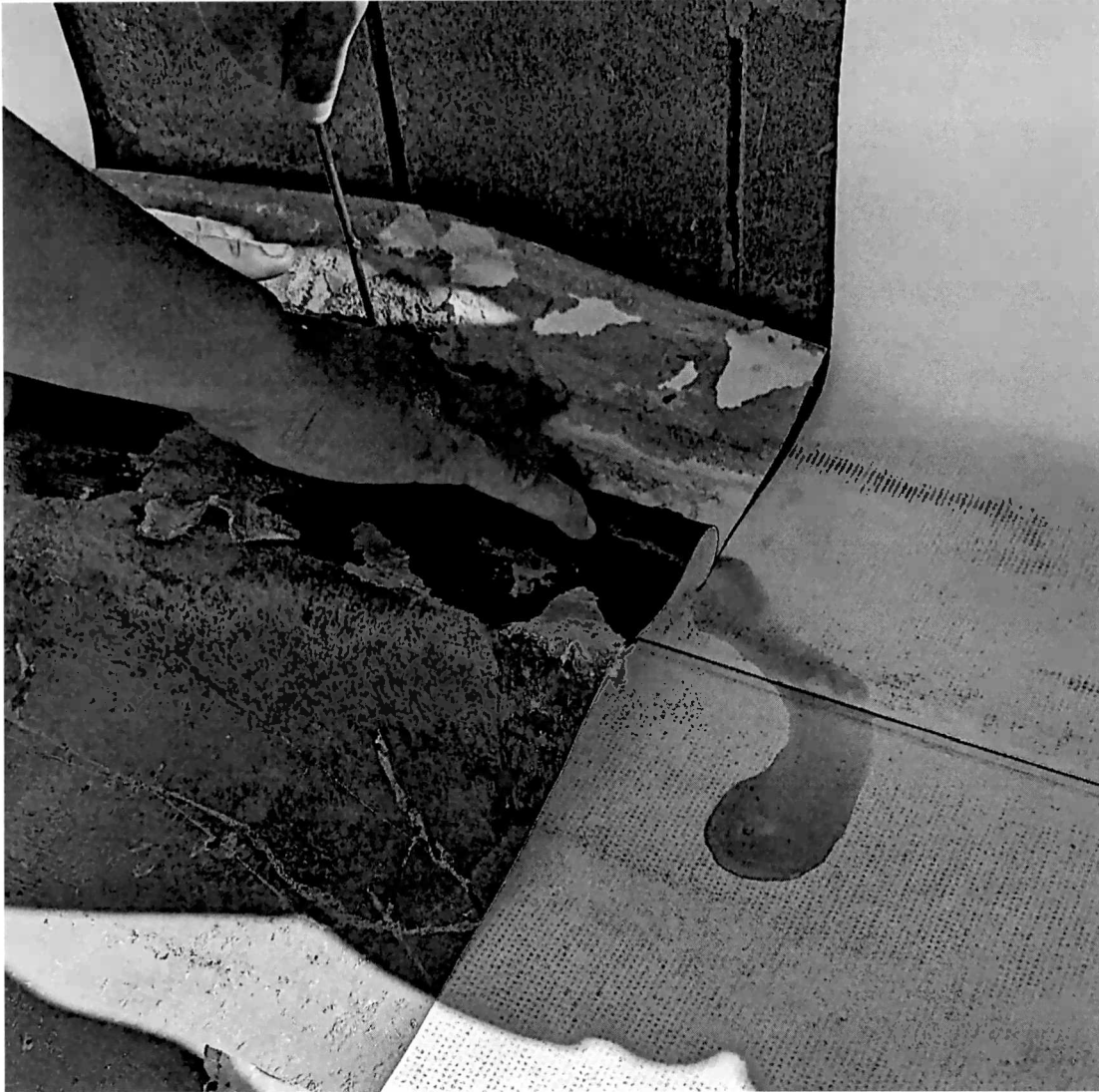
Figure 18 cut #4, when the screw was extracted the water at the screw ran off the slope. Illustration of how just how wet the roof is at the perimeter.
