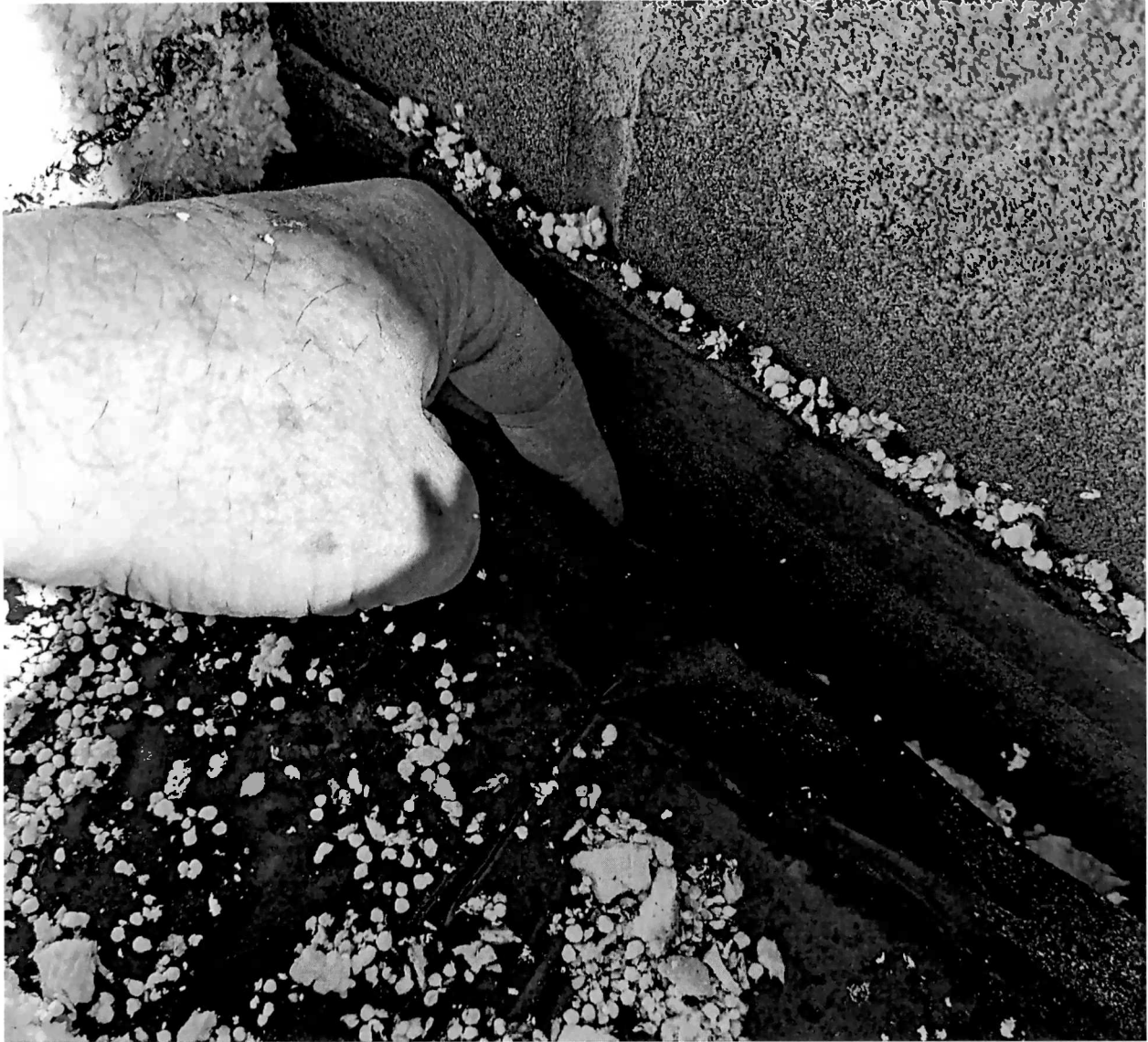
Figure 20 cut #4, the black 6-mil poly is short of reaching the wall.
