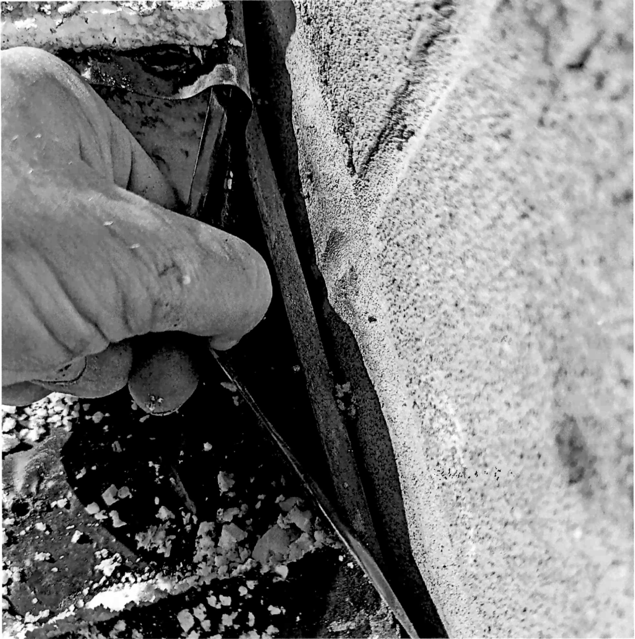
Figure 8 cut #1 pulling back the 6-mil poly reveals the angle iron that supports the deck. Below the poly is the acoustical deck. The visible block behind the angle iron was not painted with epoxy paint.
