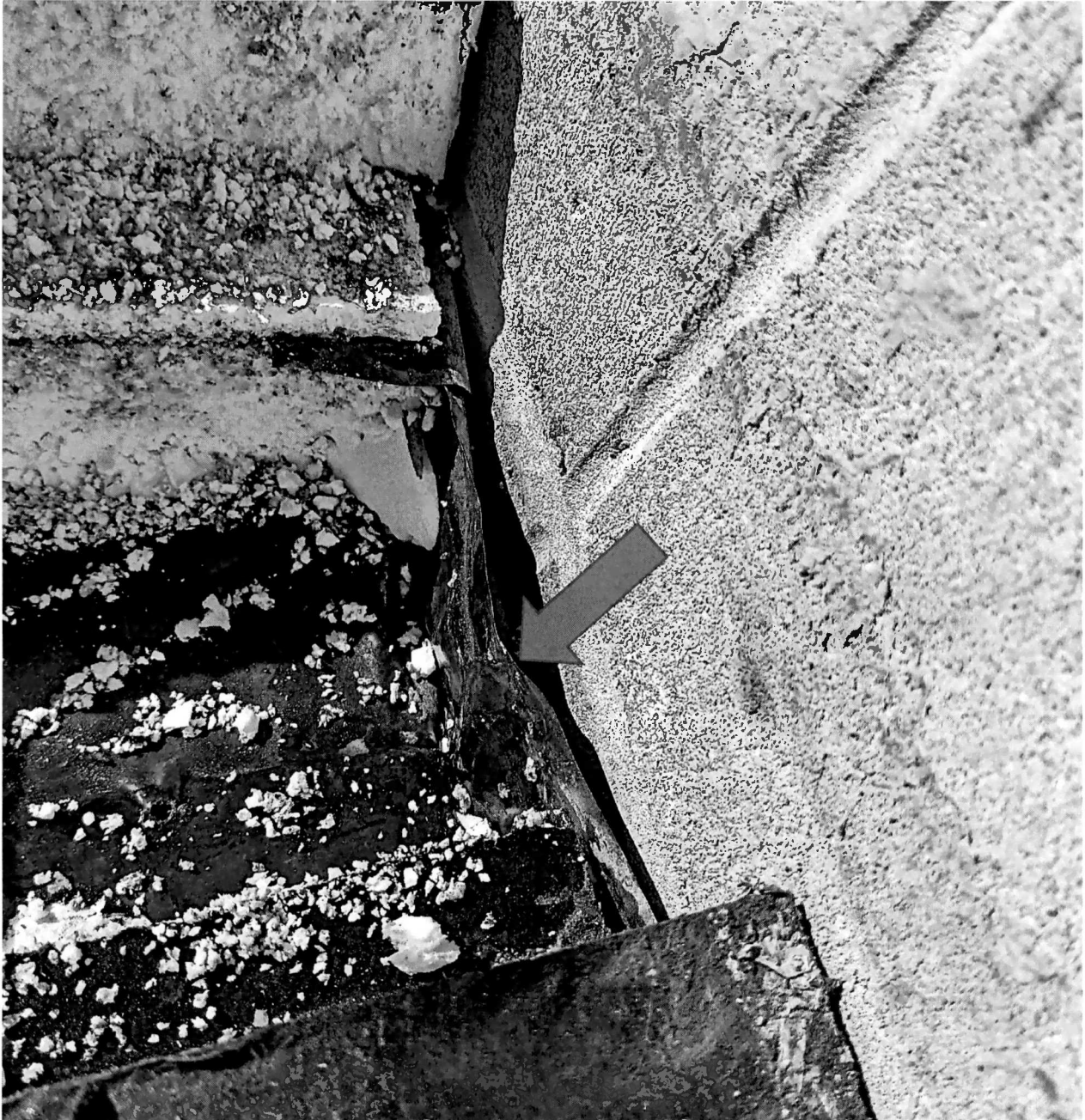
Figure 7 cut #1 below the insulation is black 6-mil polyethylene vapor barrier (arrow) that is loose laid and not sealed to the block wall. Block wall is not painted with epoxy paint like below the deck.
