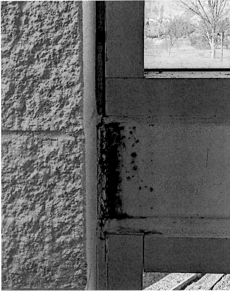
Figure 26 steel between curtain wall elements is showing signs of corrosion.
