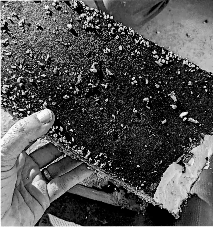
Figure 6 cut #1 second layer of 2.5-inch polyiso visible wet.
