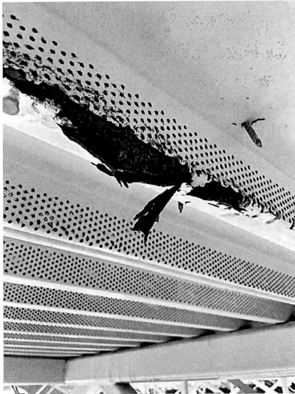
Photo-3: Severely damaged low rib of deck at north-east corner
