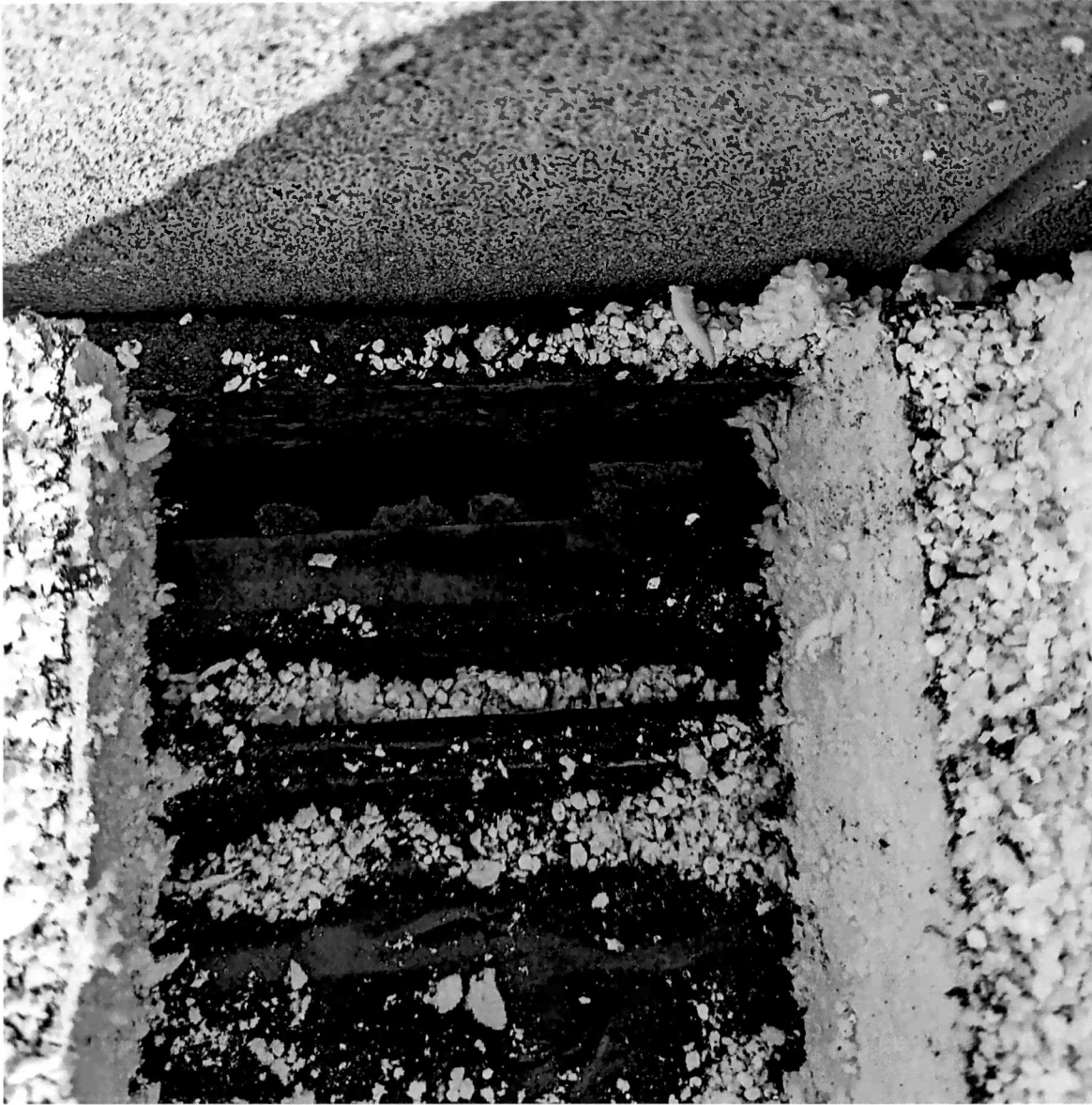
Figure 16 cut #3, below the two layers of insulation, the loose laid vapor barrier is well short of reaching the wall. The metal acoustical deck is completely corroded. The vapor barrier has sagged at the valleys of the acoustical deck.
