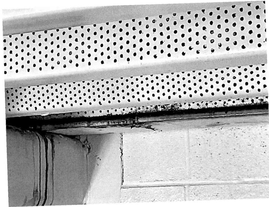
Photo-25: Severely damaged roof deck bearing at north-west wall
