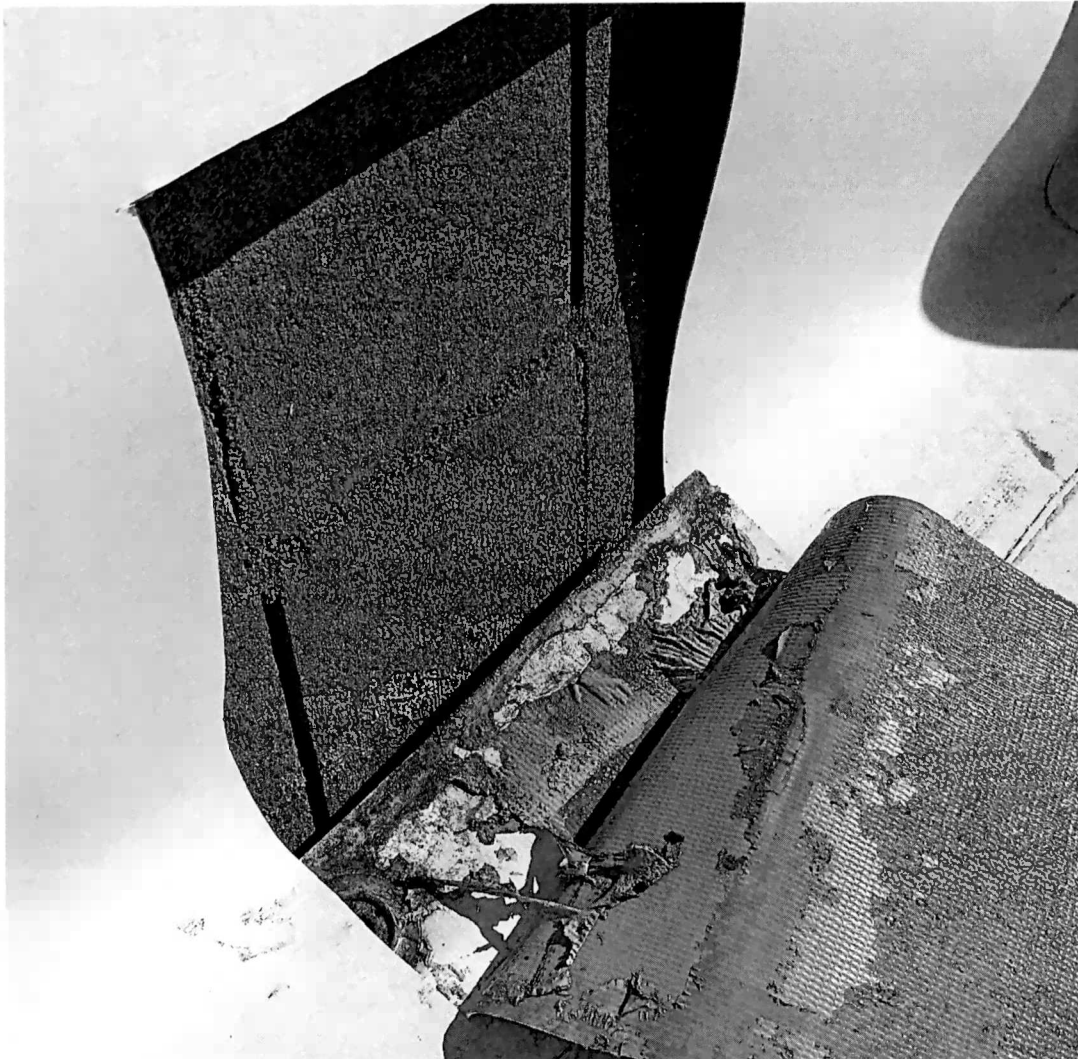
Figure 14 cut three illustrates how the roof membrane is loose and no longer attached to the block.
