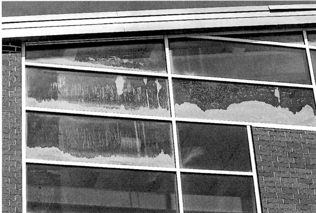
Figure 41 numerous glazed units with failed seals. Consider bringing in a Curtain Wall forensic expert before replacing any glazed units. When this many glazing unit seals fail there may be an underlying cause that if not corrected would simply result in more failures.
