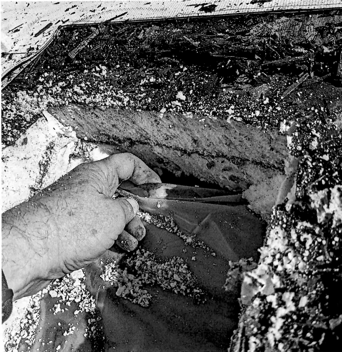
Figure 24 cut #5 below the insulation was 6-mil clear poly vapor barrier that was not attached and short of reaching to the wall vapor barrier.
