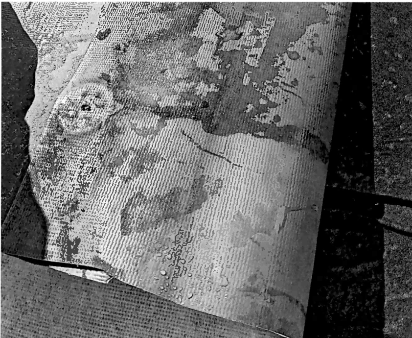
Figure 2 cut #1, Layer two, pull back show's visible beads of water below roof membrane. The top layer of the polyiso was wet to the touch.
