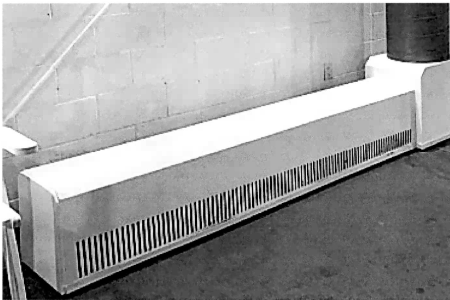
Figure 1 evacuator bench at deck level. Shown also in figure two below.
