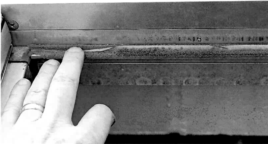
Figure 42 exterior door weather stripping appears worn.
