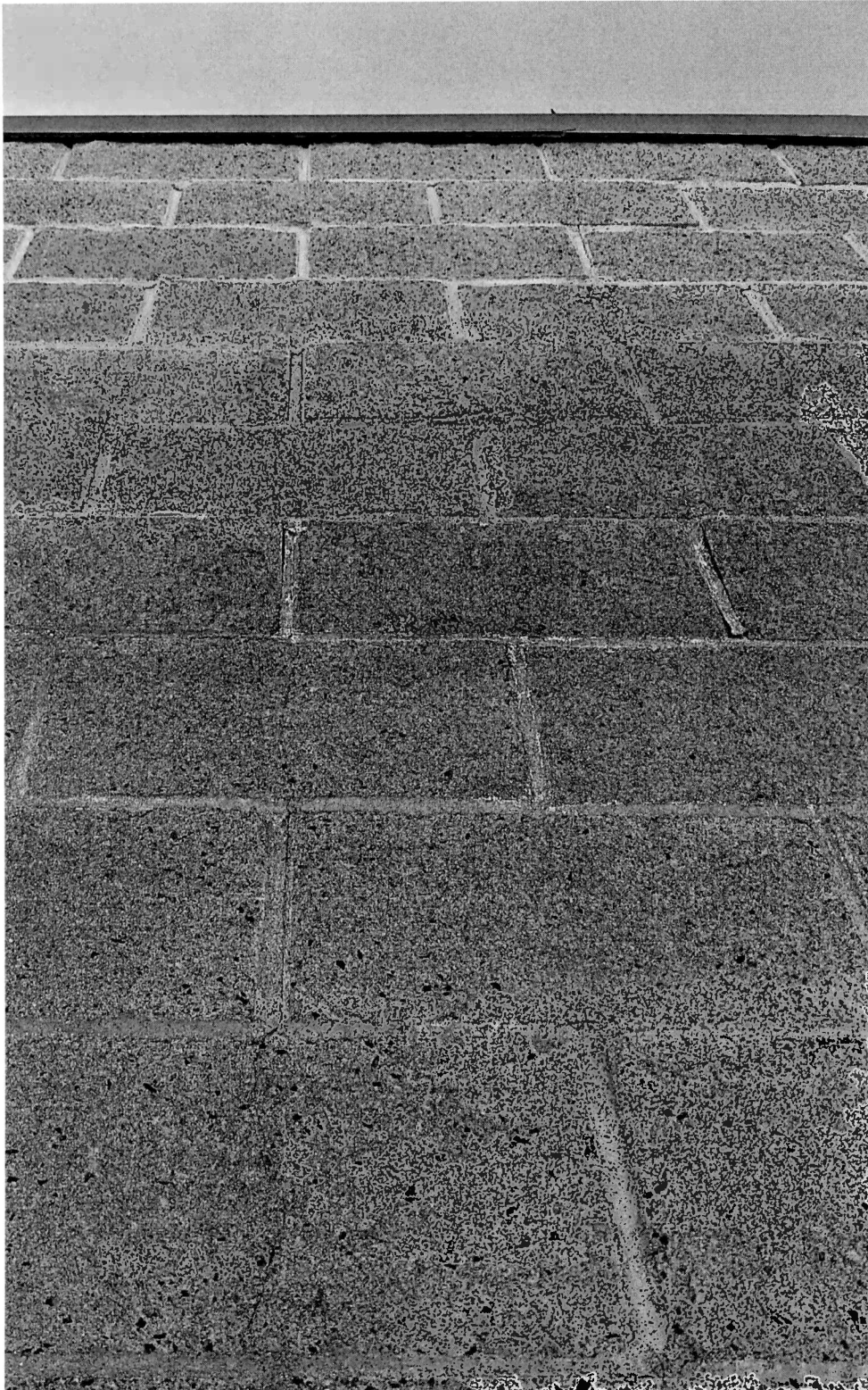
Figure 30 another photo of the North wall. The wall had no epoxy sealer on the inside surface of the block above the deck, and the roof membrane was not attached to the block. (See figure #14) There is degradation of the block joints and some discoloration of the block. The parapet block is cold and cold, but the lower block is warm on the inside and cold outside.
