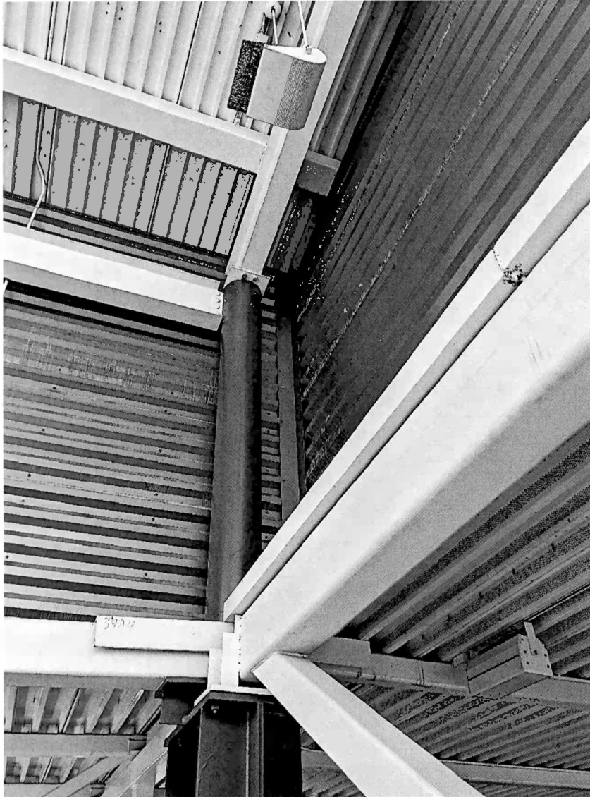
Figure 32 interior photo of the high roof. The light fixture shown is inaccessible by a lift.
