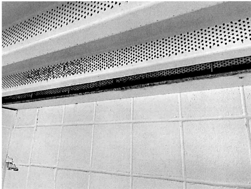
Photo-8: Severely damaged low rib of deck at north-east wall
