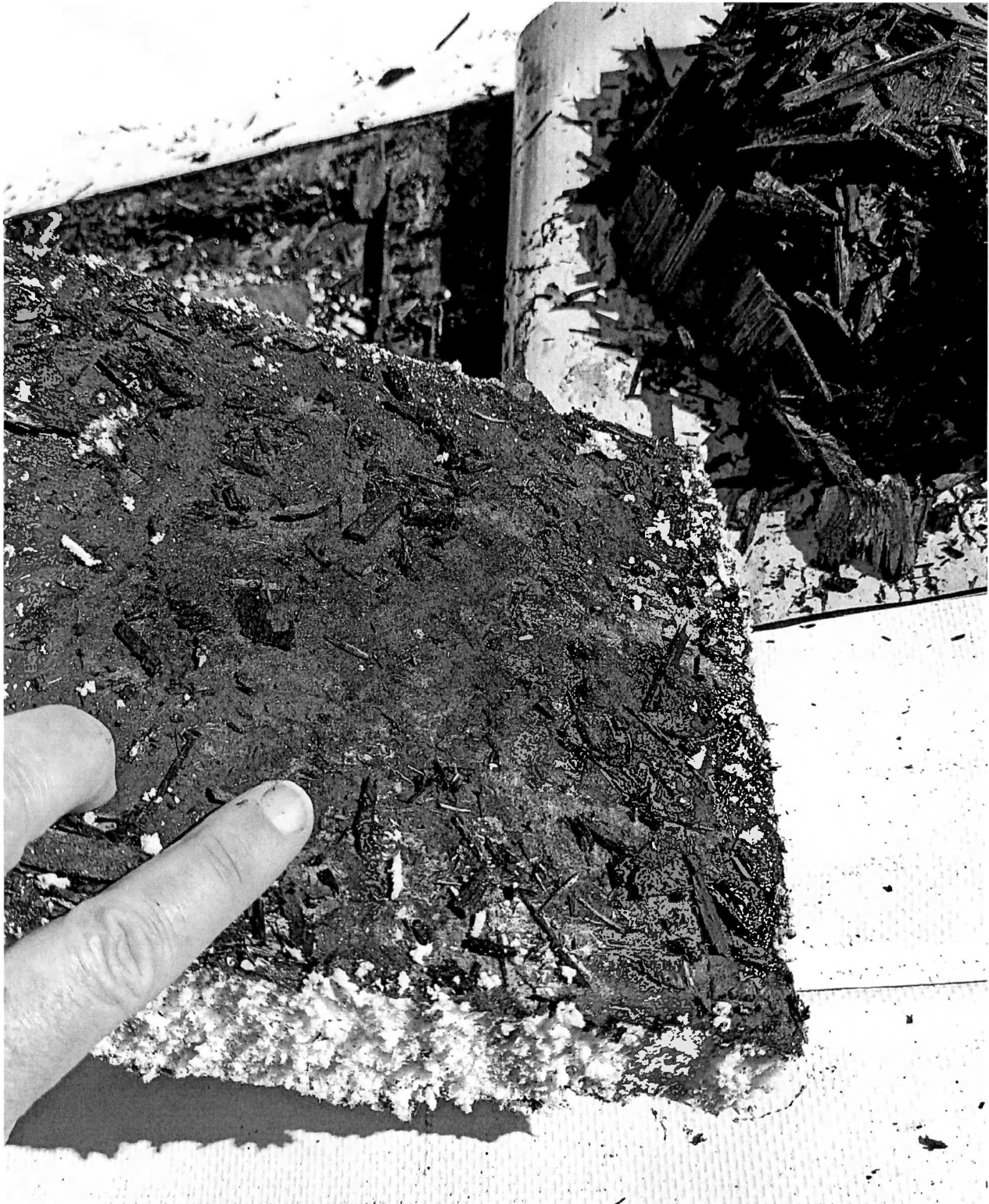
Figure 23 cut #5 below the plywood that came up in handfuls, is two layers of 2-inch polyiso insulation.
