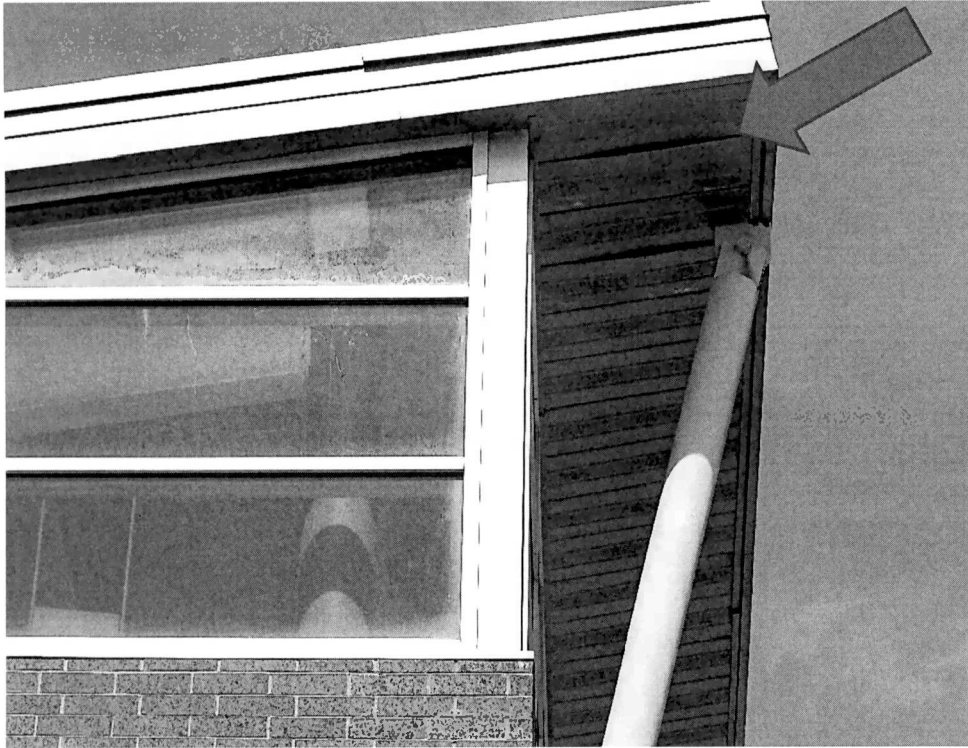
Figure 40 high roof south exposure, there appears to be damage to the soffit. This might be due to an ice or wind load.
