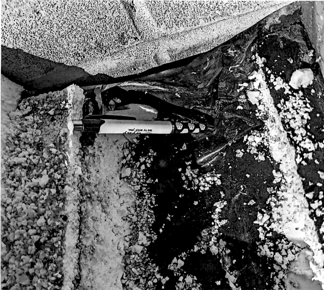
Figure 9 cut #1 the screw fastener at this location (pen) was in the valley of the deck and probably did not have a seal at the penetration. Screws that hit the ridge seal a bit better because of the backing of the deck.
