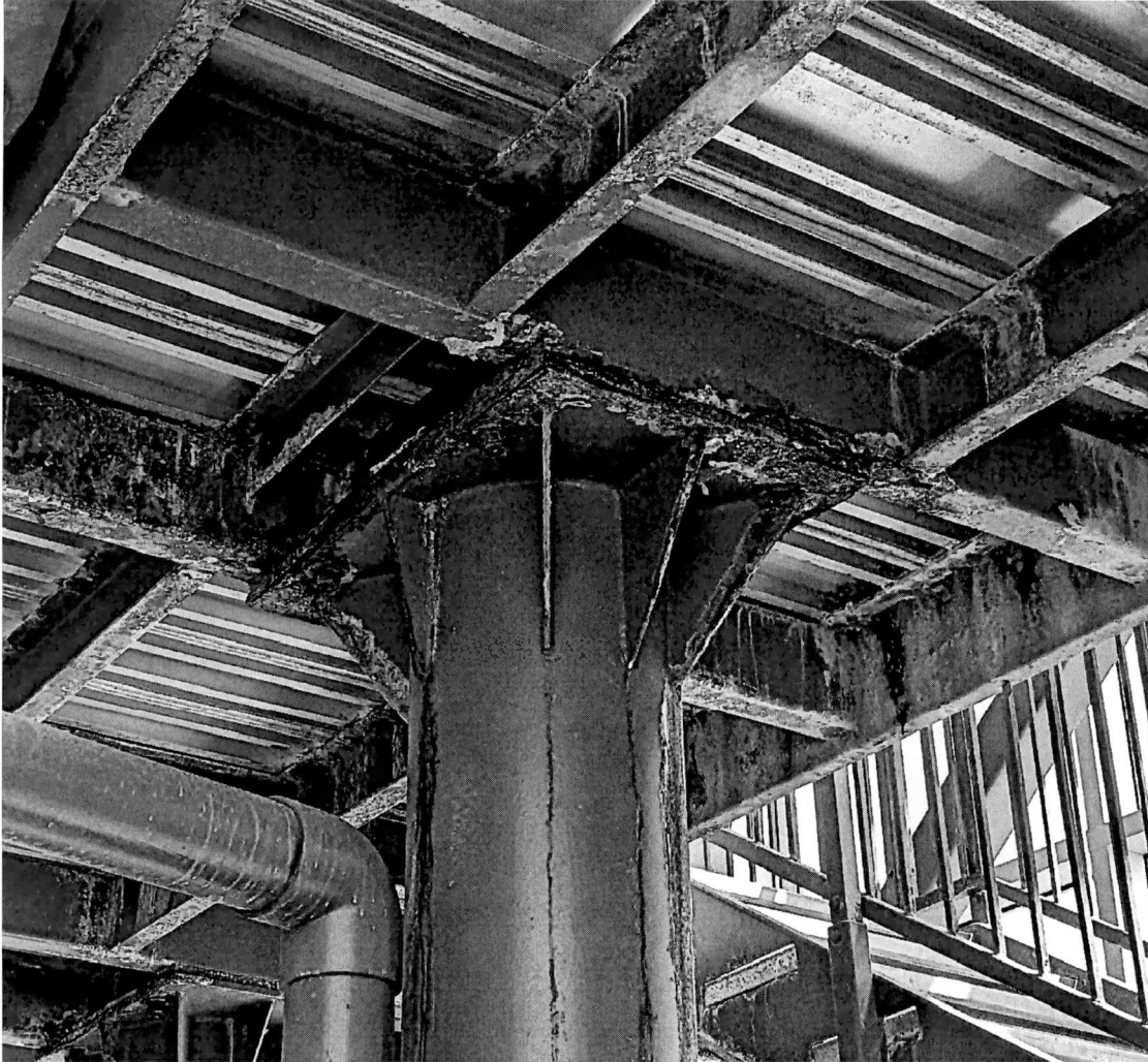
Figure 27 significant corrosion of the column top of the slide. This corrosion is extreme and has damaged the structure. This damage should be investigated immediately to determine the safety of the assembly.
