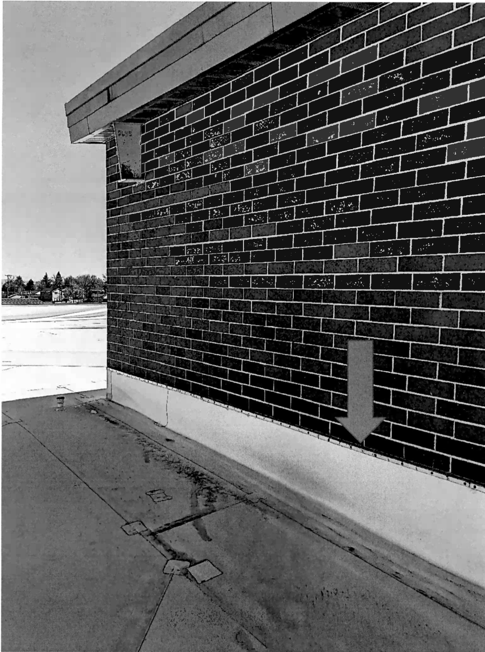
Figure 33 North face brick at stair tower. Note no thru flashing at the term bar (arrow). Also note the sagging roof membrane that is not adhered any longer. A wrap on the membrane with my knuckles, below the term bar indicated a solid backing like brick.
