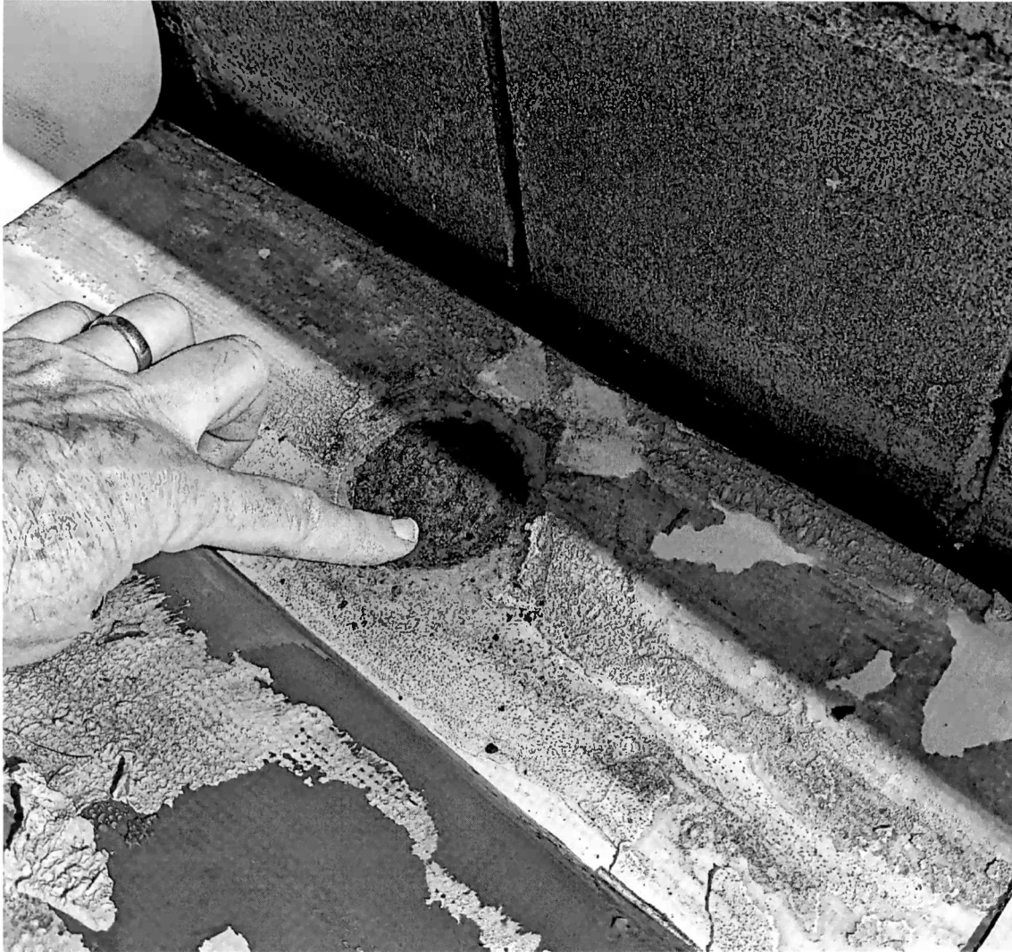
Figure 17 cut #4, all the cuts were wet below the first layer, but this shows a small pond at the washer for the screw.
