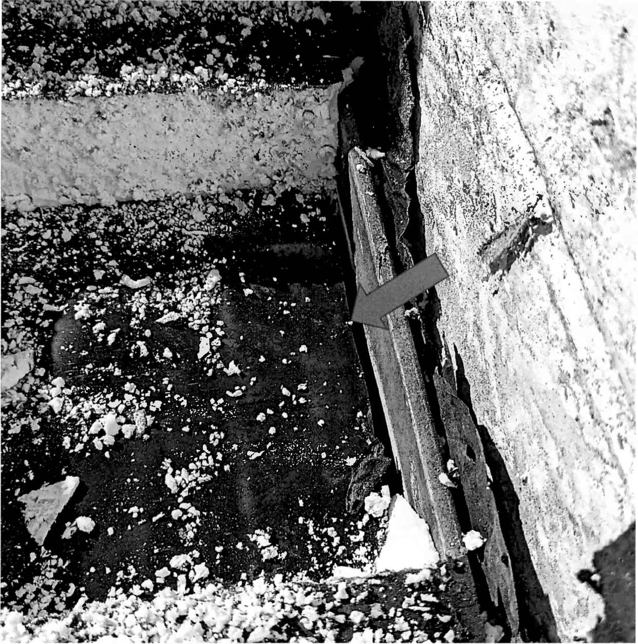
Figure 13 below the two layers of insulation (wet) is the black vapor barrier that is 1/2 inches short of angle iron and 1.5 inches short of meeting the wall (arrow). The paper from the back of the sheet rock is also visible.
