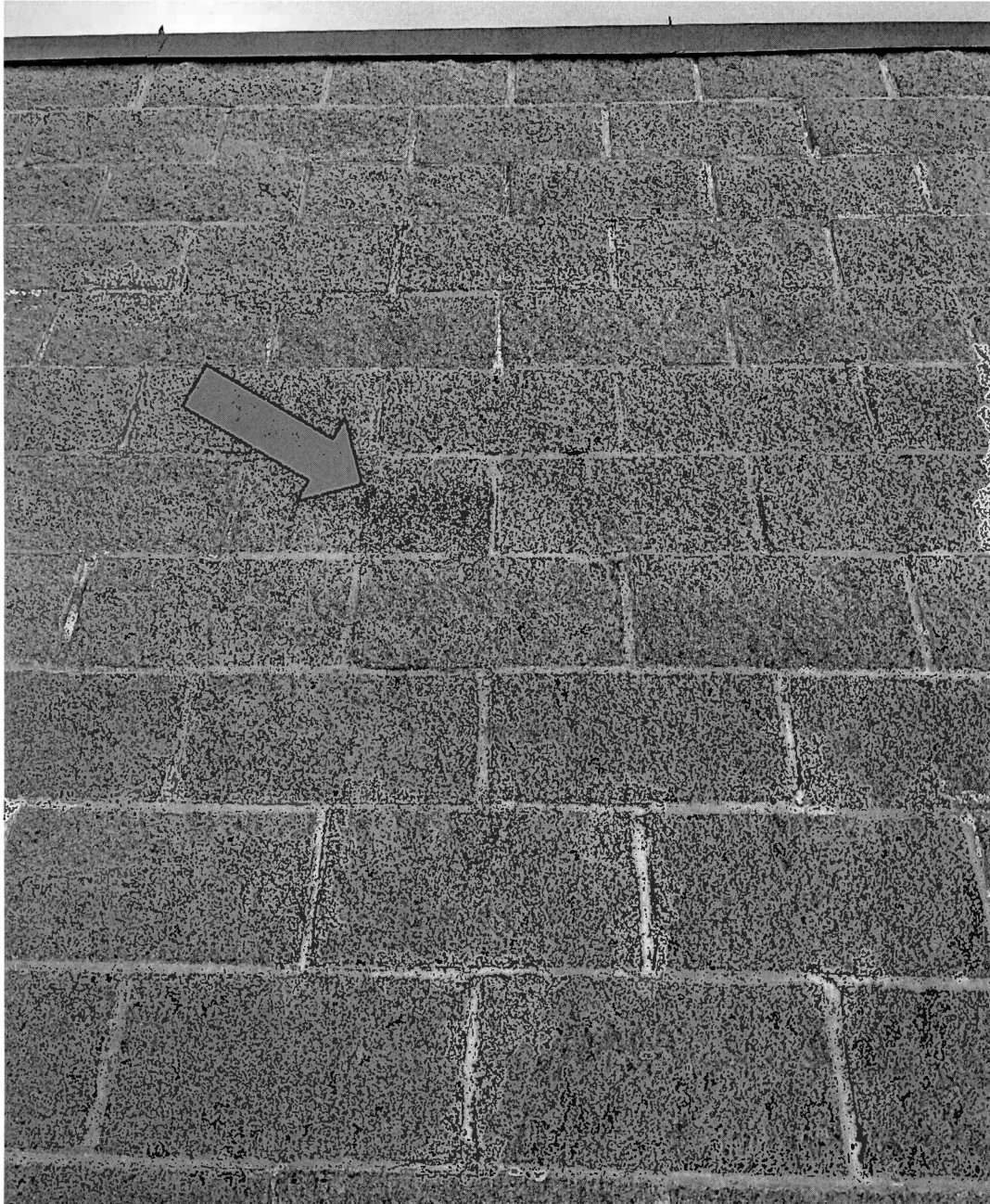
Figure 29 North wall just left of the attached ladder. There is a small amount of spalling (arrow) This is occurring at an elevation that coincides roughly with where the roof connects to the parapet. There are also signs of efflorescence indicating regular wetting of the wall from the inside.
