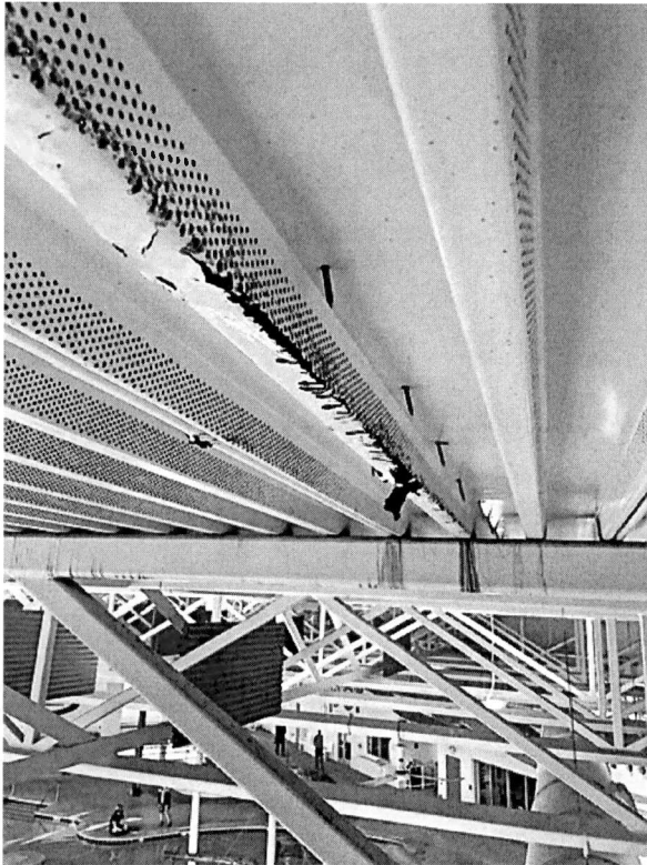
Photo-1: Severely damaged low rib of deck at north-east corner
