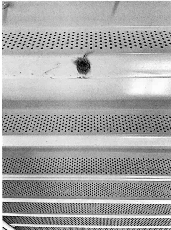
Photo-4: Low rib test location with bare steel exposed
